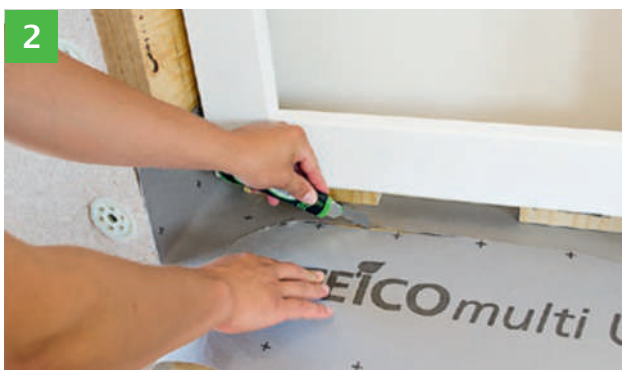
2 The windows are installed on the membrane. Before STEICOfix is installed, the sheet is cut back „half-moon-shaped“ (see Fig. 5).
