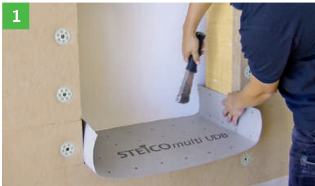
1 Attachment of STEICOmuli UDB (diffusion-open membrane) as temporary weather protection until window installation.
